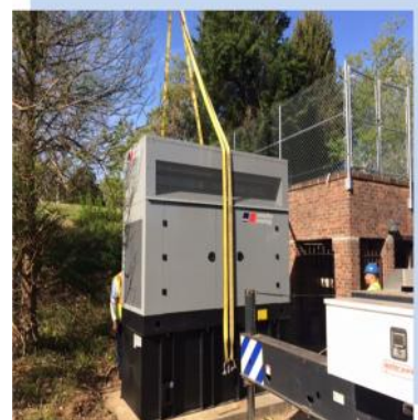
MetCom staff lowering a replacement generator at the St. Mary's City Wastewater Pumping Station
