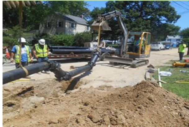
Patuxent Park Water & Sewer Replacement and Rehabilitation Project: Phase 3 Water Line Replacement
