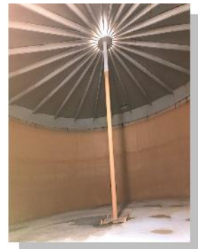
(Right Photo) Interior of the Piney Point Landings Water Storage Tank during the medi-blasting process
