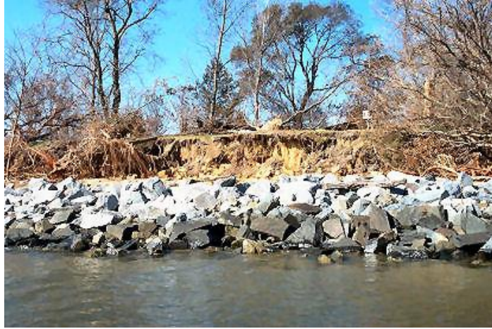
Source: Bank erosion due to vertical expansion of zone of wave influence. St. Clements I., Potomac R., St. Mary's Co. - S. Alexander (photographer), 2003, St. Mary's Co. Dept. of Public Works
